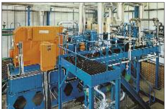
Steam Turbine Gerator Set. Coupling fitted between the gearbox and alternator.
