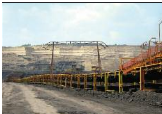
Conveyor. Couplings fitted on the input and output on conveyor drives.
